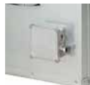
Outside connecting box and base stands
